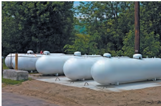
Photo 7.3 Cylindrical pressure vessels.
