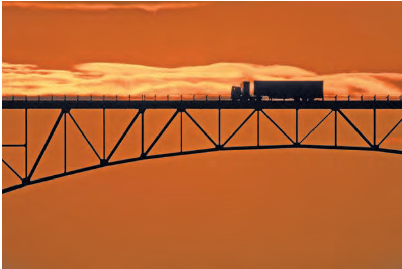
Photo 1.1 This bridge truss consists of two-force members that may be in tension or in compression.
